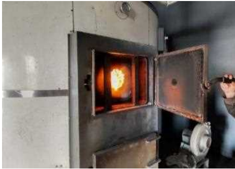
An existing coal-fired boiler (food factory for convenience stores)
